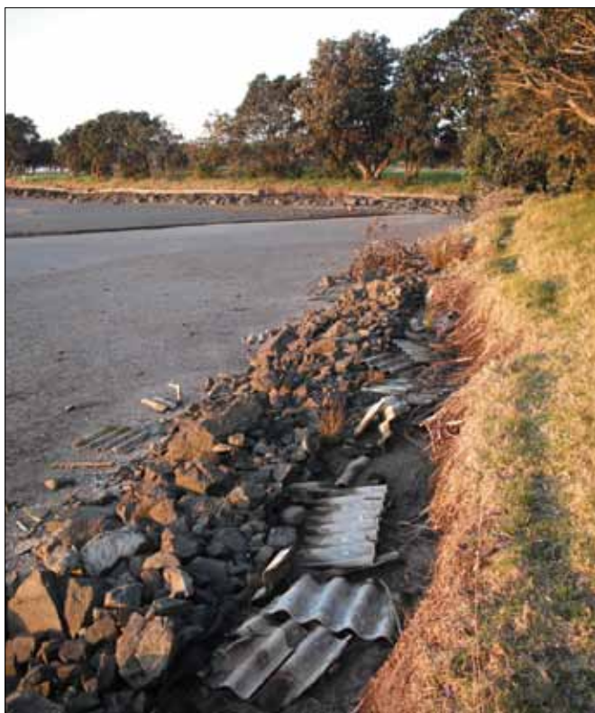
Exposed metal and asbestos as old Seawall breaks up.
